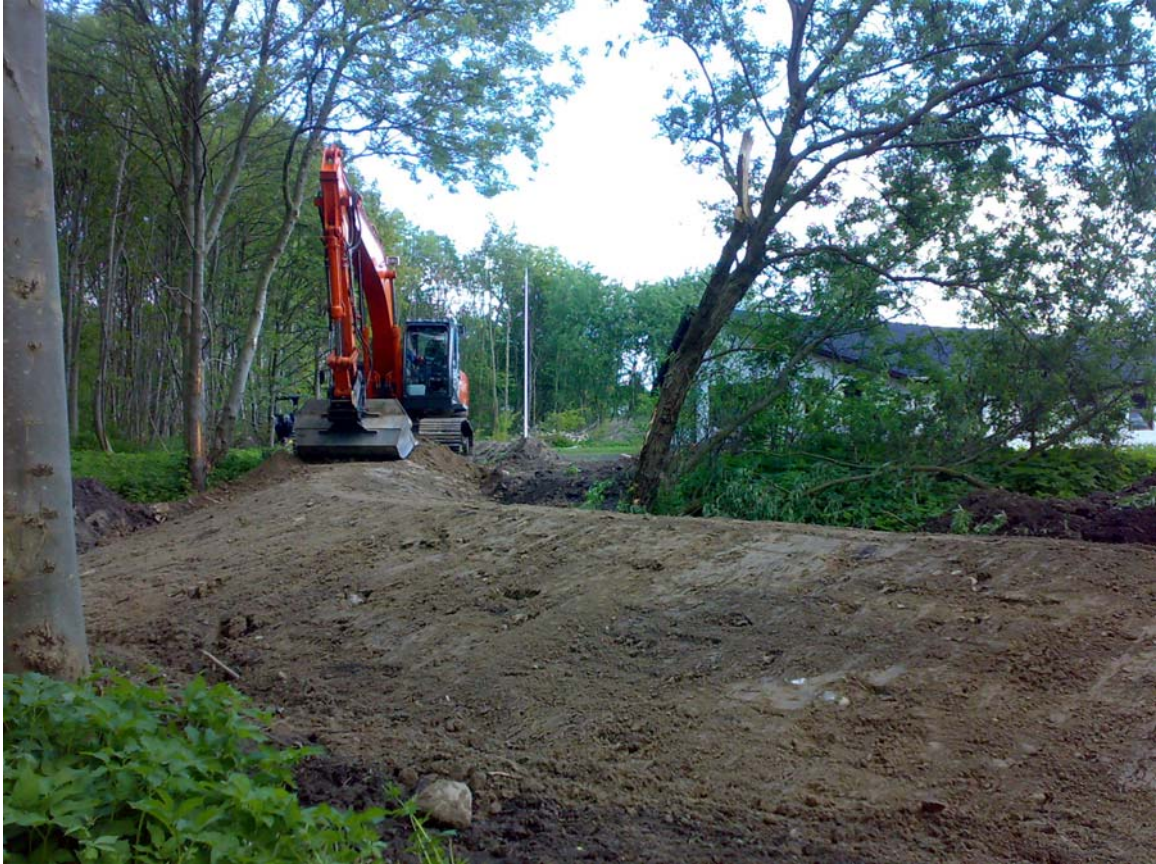
Figure 4 Example of adaption measures in Greve. Due to the flooding in 2007, a barrier along a stream has been build to prevent future flooding. Photo: Greve municipality
