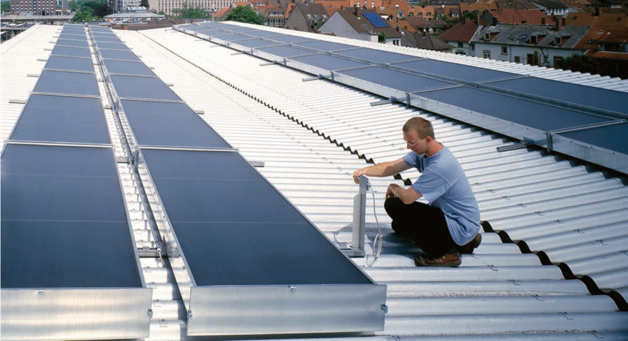
Sun-panels produce electricity in Freiburg. Photo: Institution of Civil Engineers, www.ice.org.uk
