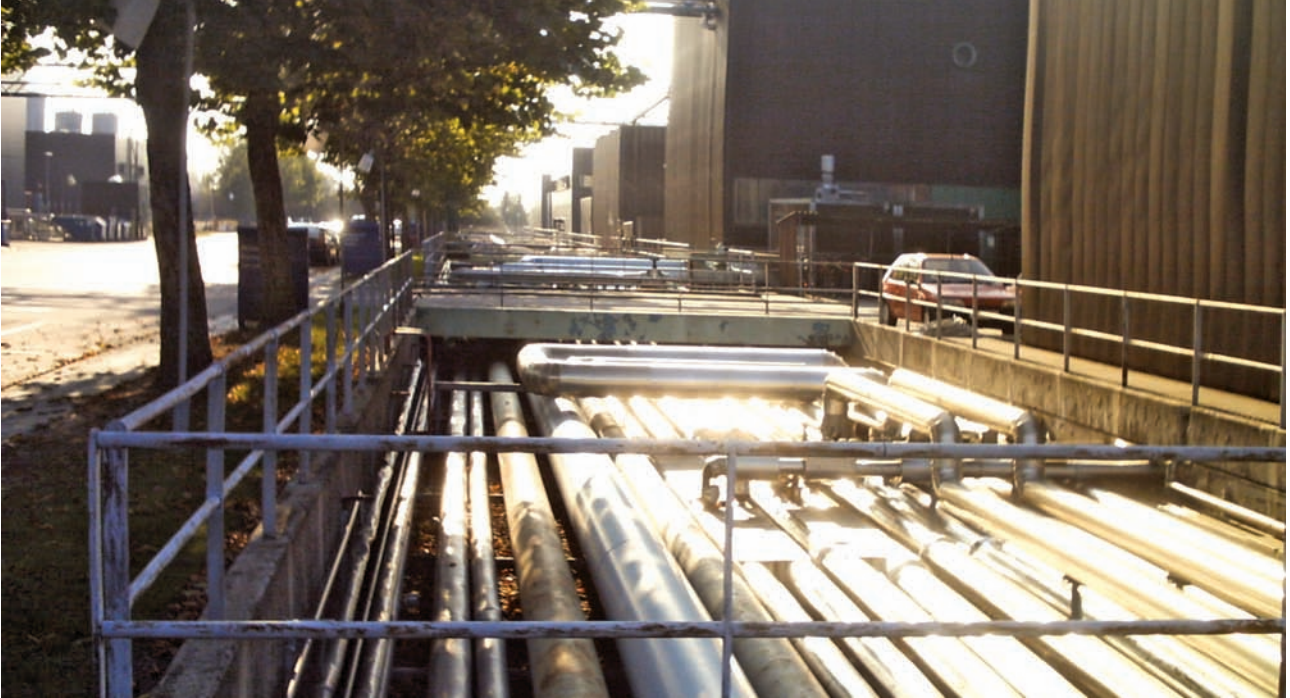
Piping at the Industrial Symbiosis plant in Kalundborg. Photo: Rasmus Ole Rasmussen
